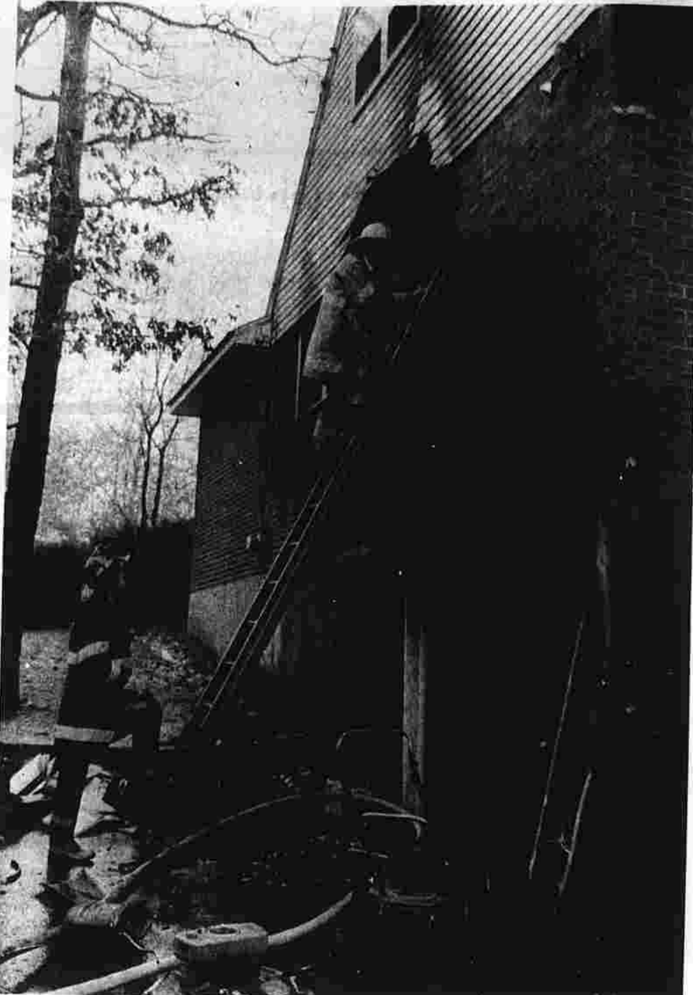
Manchester Deputy Fire Chief Roy Stratton, top of ladder, inspects fire damage to a house at 166 Ludlow Road, Manchester. Firefighters responded to the scene late Thursday afternoon and were recalled early this morning when the blaze rekindled. The interior of the home was heavily damaged and one person was injured in the fire. (Herald photo by Pinto)
